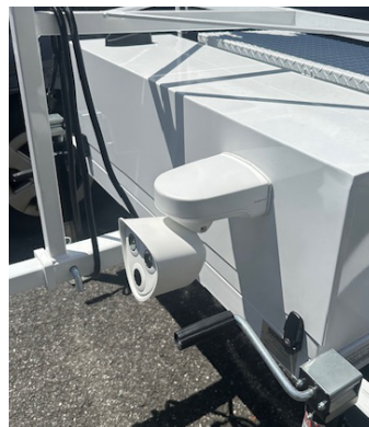
Camera mounted to battery box
