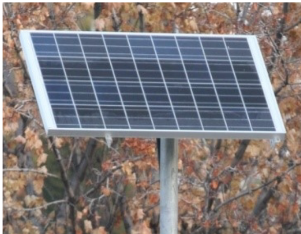
Figure 6, Larger solar panel
